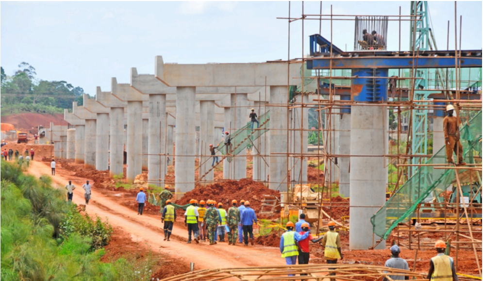
Construction site for the expansion of the Northern by pass highway. In Uganda, the rush for land for direct foreign investment and industrialization has informed the manifest colossal investment in infrastructure development including airports (both new and expansion of the existent ones), roads across the country, railway (through the Standard Gauge Railway project) etc. This calls for compulsory land acquisition, the quest of this research.
